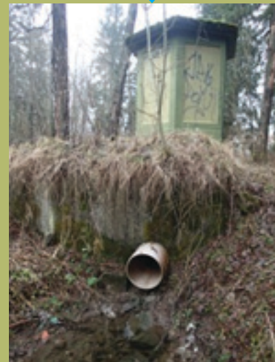
Combined Sewer Overflow (CSO)
